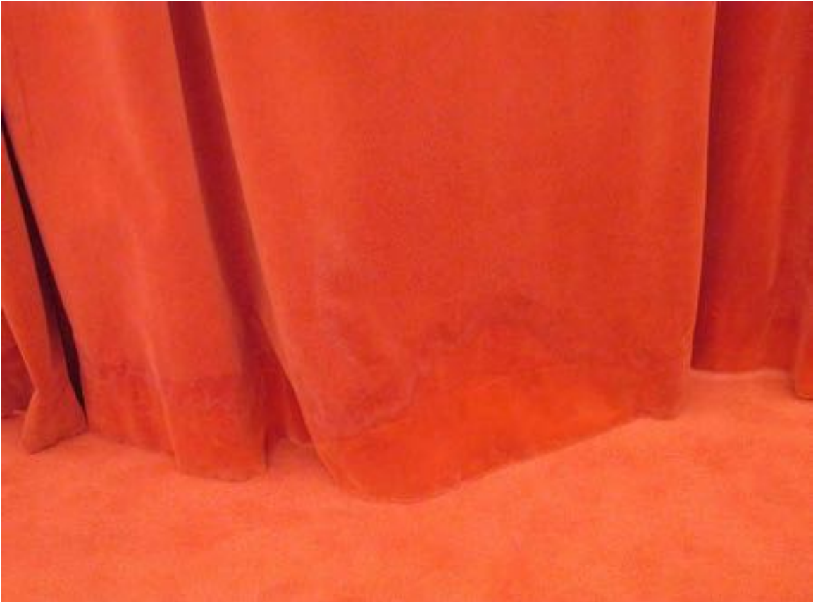
Figure 10-186 - Typical water staining on curtains in the Pavilion, 2015 (Harboe Architects).
