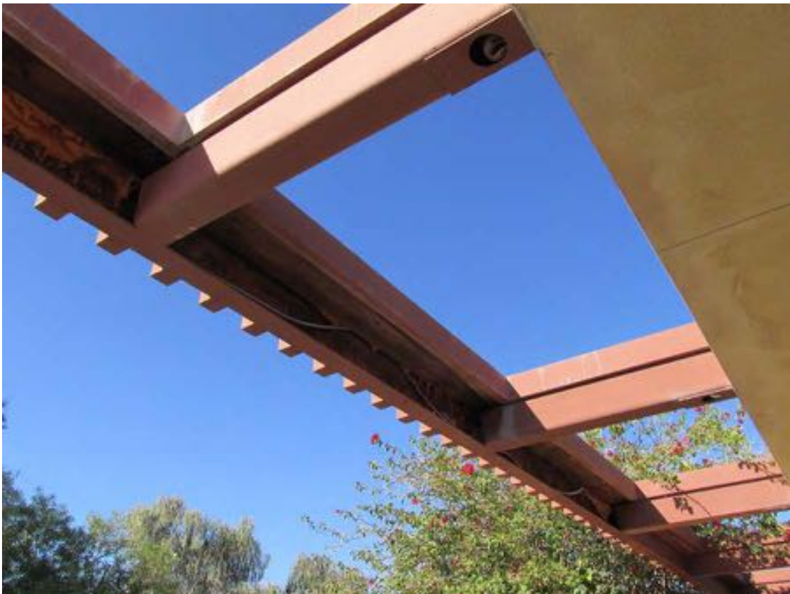
Figure 10-237 - Missing fascia on back of trellis on south side of Finance Office (Harboe Architects).
