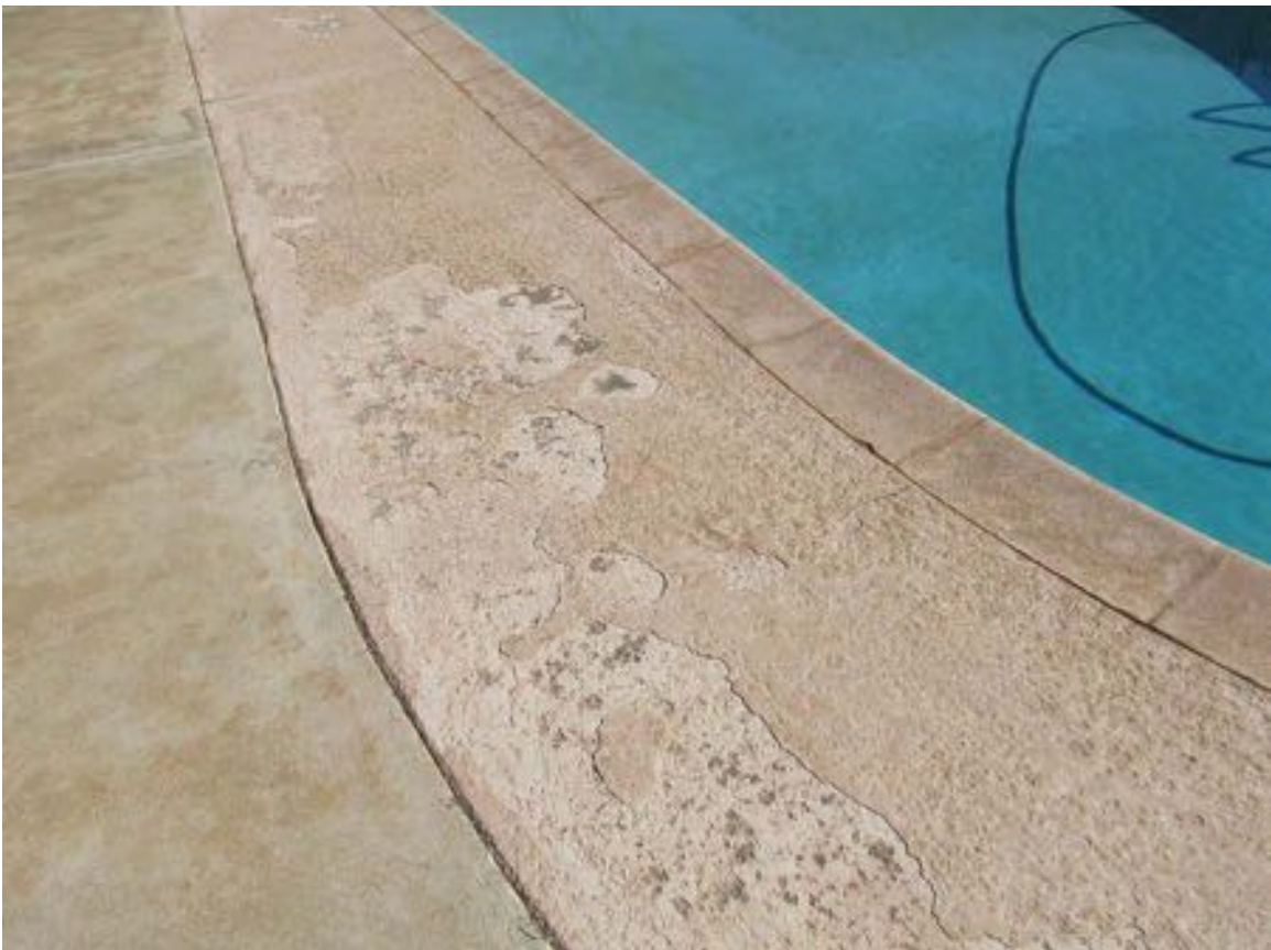
Figure 10-132 - Delaminated mortar topping of inner pool deck, 2015 (Harboe Architects).
