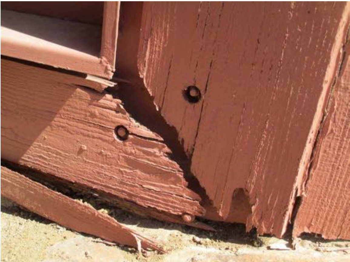
Figure 10-18 - Damaged wood on south side of Drafting Studio, 2014 (Harboe Architects).
