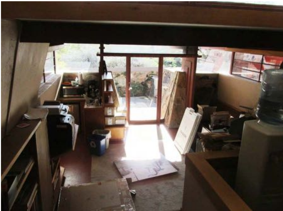
Figure 11-212 - Interior of Dr. Joe Office looking east at lower level, 2015 (Harboe Architects).
