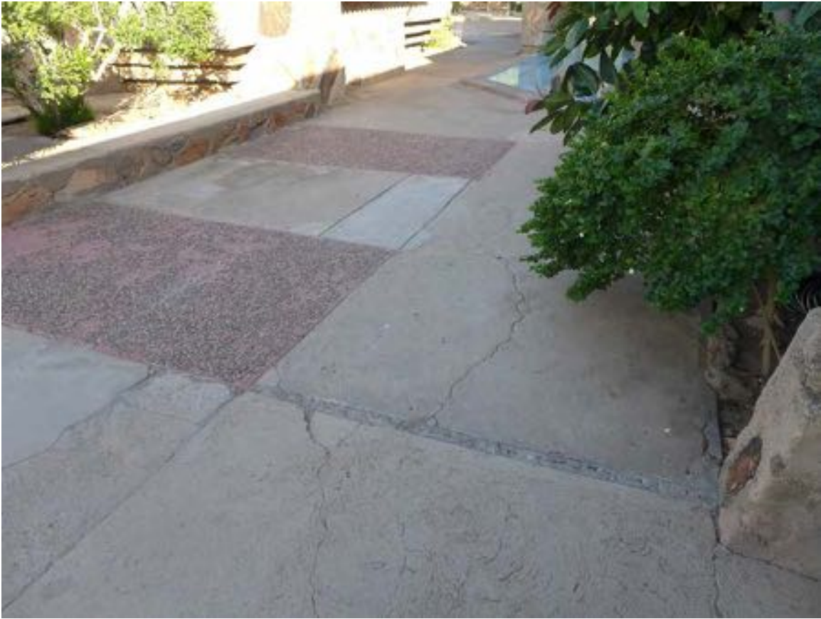
Figure 11-253 - Damaged concrete paving on north side of living quarters, 2014 (Harboe Architects).
