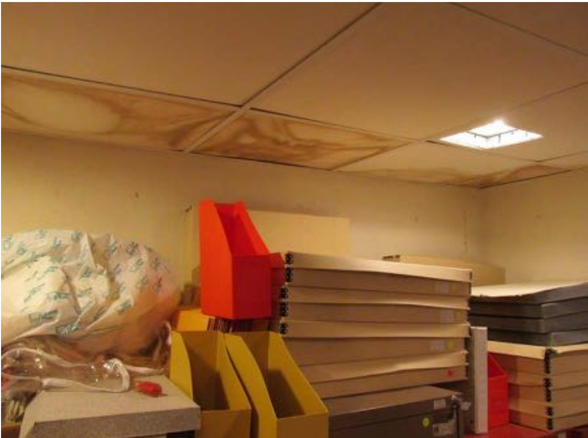
Figure 10-205 - Water damaged ceiling tiles in the reference book room, 2015 (Harboe Architects).
