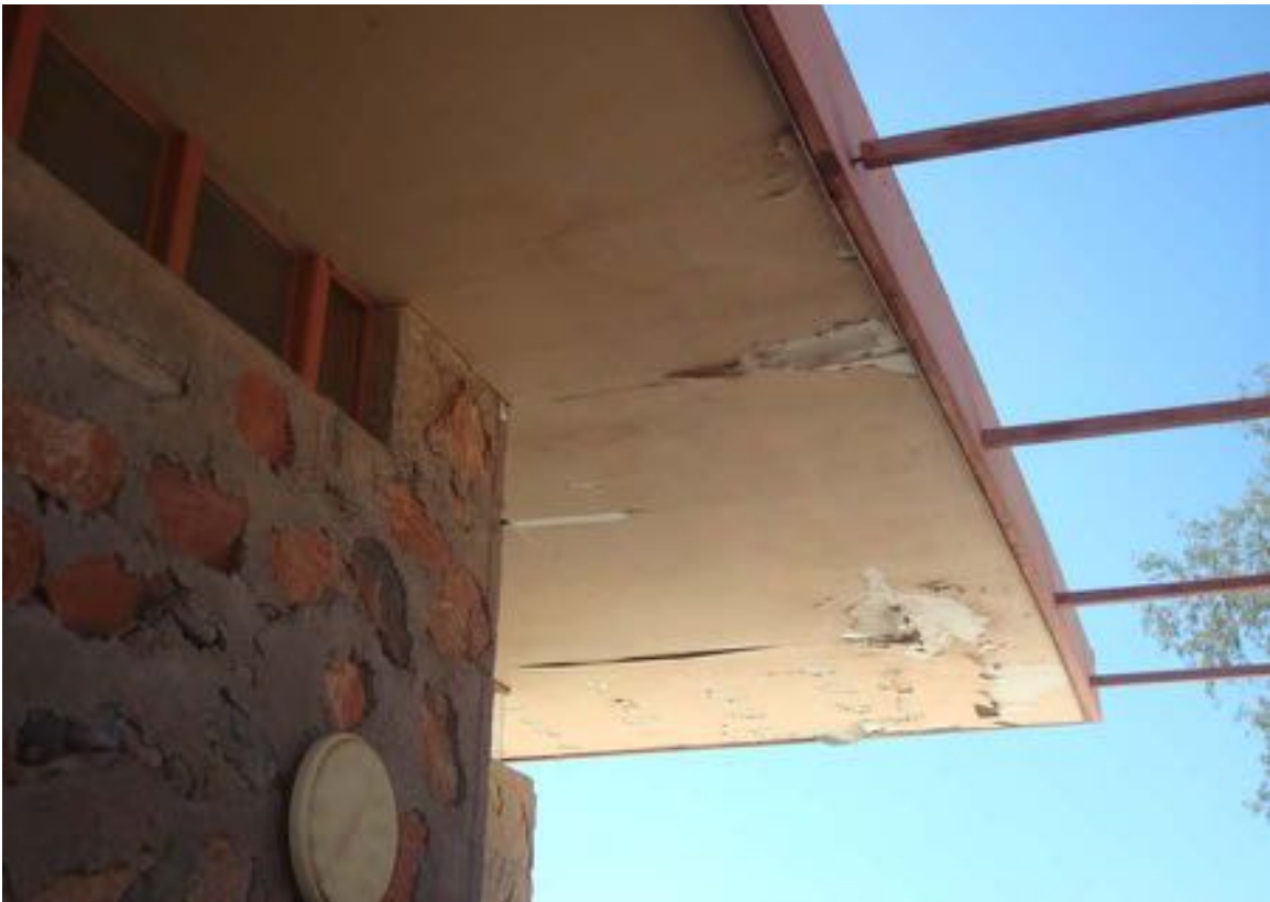
Figure 11-232 - Damage to soffit on Tower Office, 2015 (Harboe Architects).
