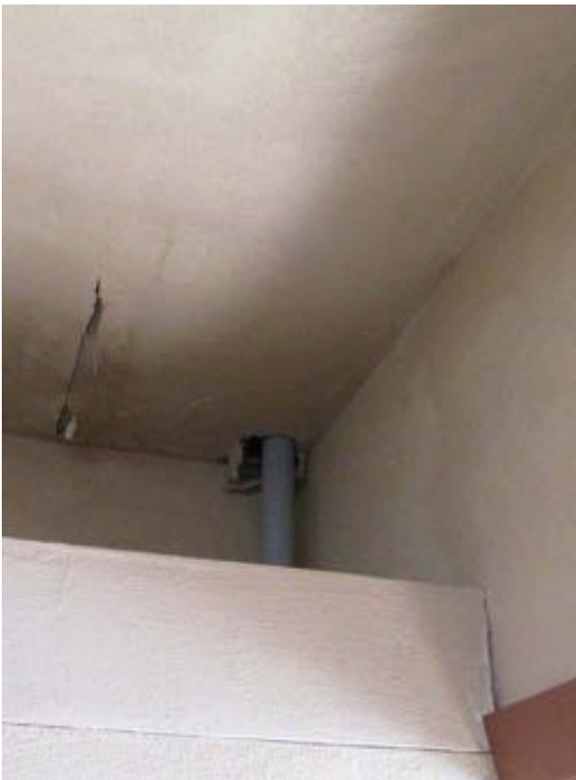
Figure 10-218 - Water damage at kitchen ceiling, 2015 (Harboe Architects).
