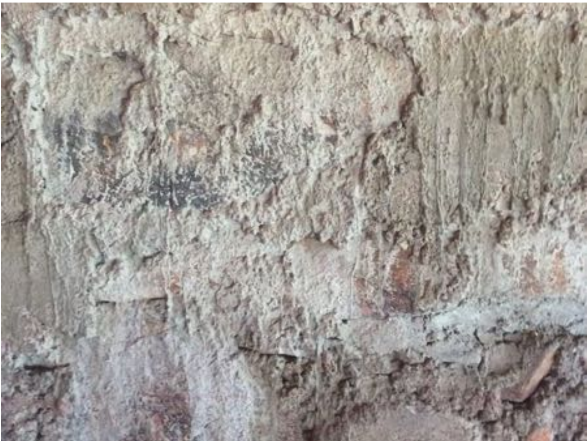
Figure 10-42 - Water damage on desert masonry wall, 2014 (Harboe Architects).
