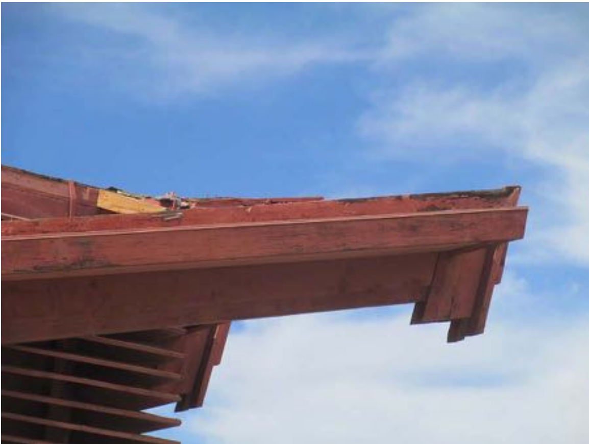
Figure 11-91 - Detail of Water Tower roof showing damaged wood, 2014 (Harboe Architects).
