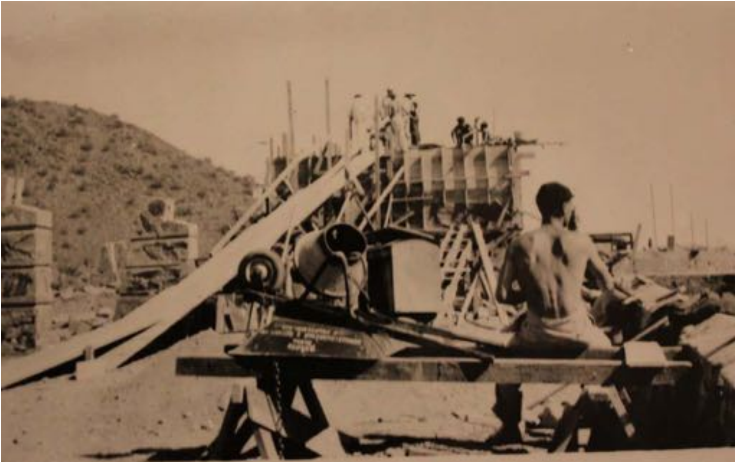
Figure 6-12 - Construction of Kitchen and Drafting Studio, ca 1938 (The Frank Lloyd Wright Foundation Archives, The Museum of Modern Art | Avery Architectural & Fine Arts Library, Columbia University, New York).
