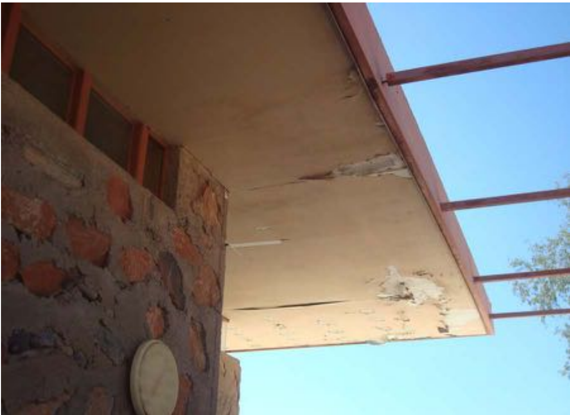
Figure 10-288 - Damage to soffit on Tower Office, 2015 (Harboe Architects).
