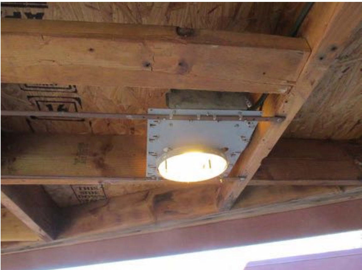
Figure 10-159 - Soffit on north side with exposed wood structure and deck, 2015 (Harboe Architects).
