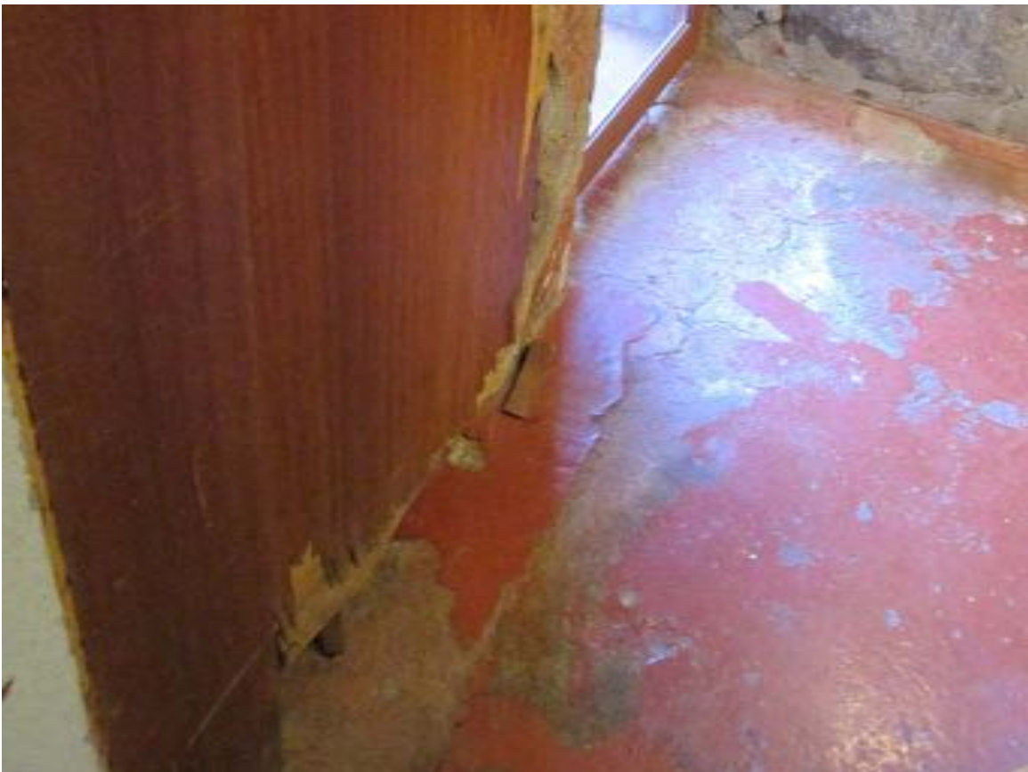
Figure 10-86 - Damaged wood veneer door and painted floor in the hallway outside the kitchen, 2015 (Harboe Architects).
