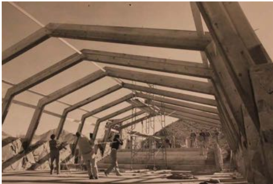
Figure 7-83 - Construction of the Pavilion ca. 1955 (The Frank Lloyd Wright Foundation Archives, The Museum of Modern Art | Avery Architectural & Fine Arts Library, Columbia University, New York).
