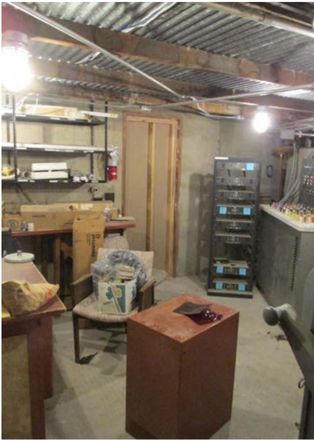
Figure 10-188 - Electrical room, 2015 (Harboe Architects).
