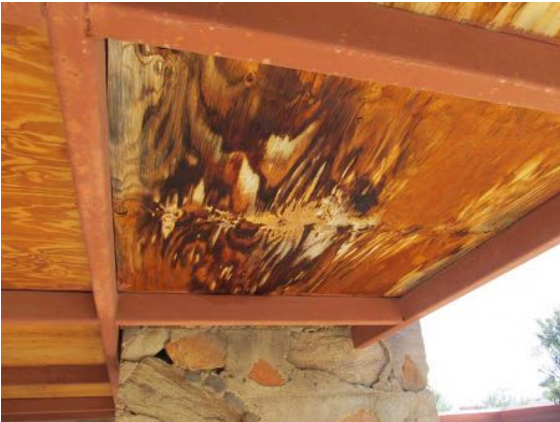
Figure 10-125 - Damaged underside of roof decking at Apprentice Court, 2015 (Harboe Architects).
