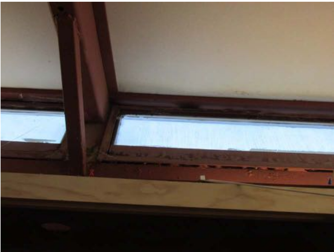
Figure 10-213 - Clerestory windows showing corrosion on metal frame, 2014 (Harboe Architects).
