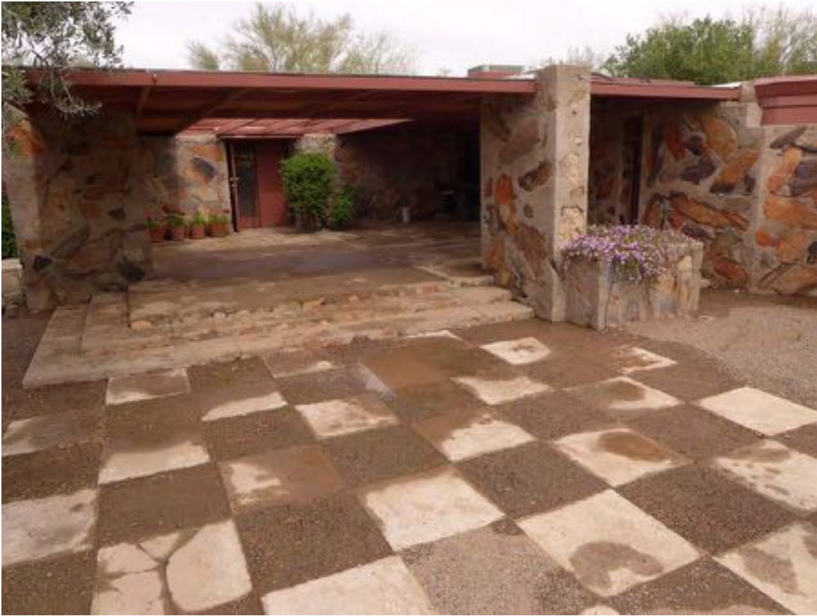
Figure 10-315 - Apprentice Court showing damaged pavers, 2014 (Harboe Architects).
