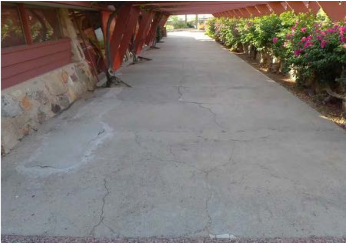
Figure 10-314 - Damaged concrete paving on north side of Studio, 2014 (Harboe Architects).
