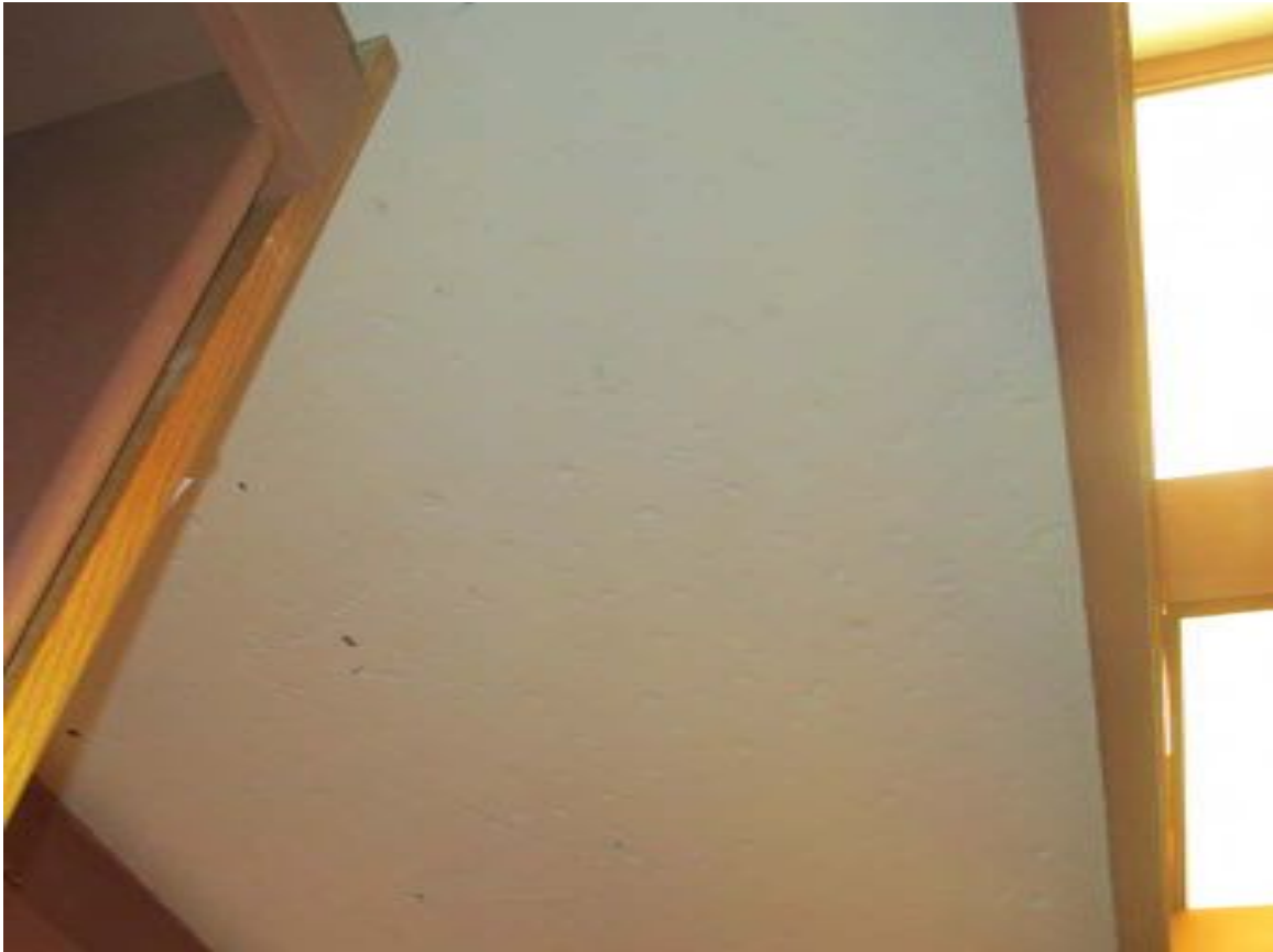
Figure 10-31 - Damaged kitchen ceiling, 2014 (Harboe Architects).
