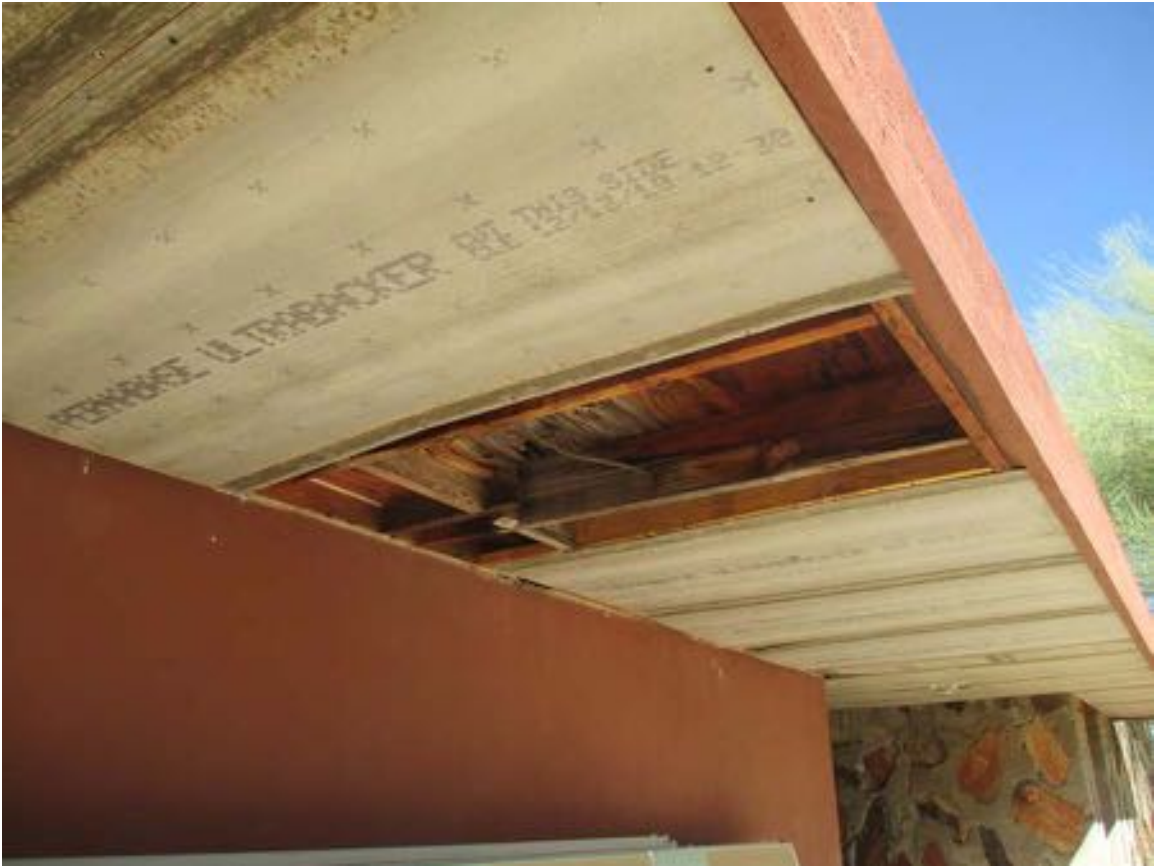
Figure 10-180 - Damaged soffit under flat roof on east side of the Pavilion, 2014 (Harboe Architects).
