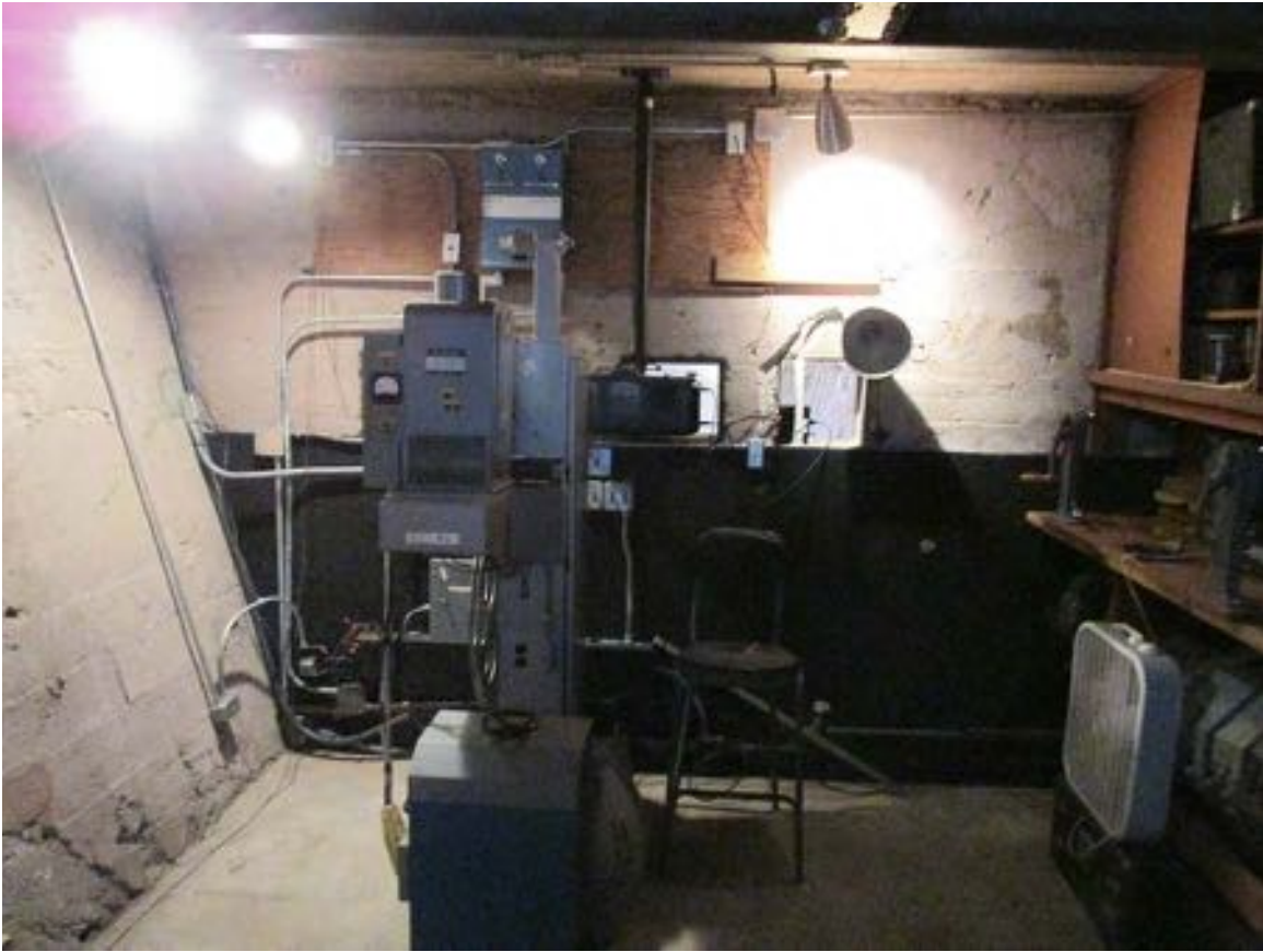
Figure 10-102 - Cabaret projection room, 2015 (Harboe Architects).
