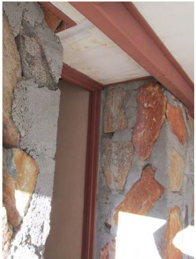
Figure 10-219 - Water staining on canvas ceiling next to kitchen entrance, 2015 (Harboe Architects).
