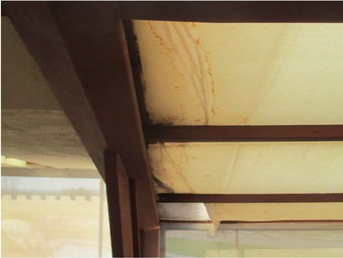
Figure 10-25 - Damaged canvas roof, 2014 (Harboe Architects).
