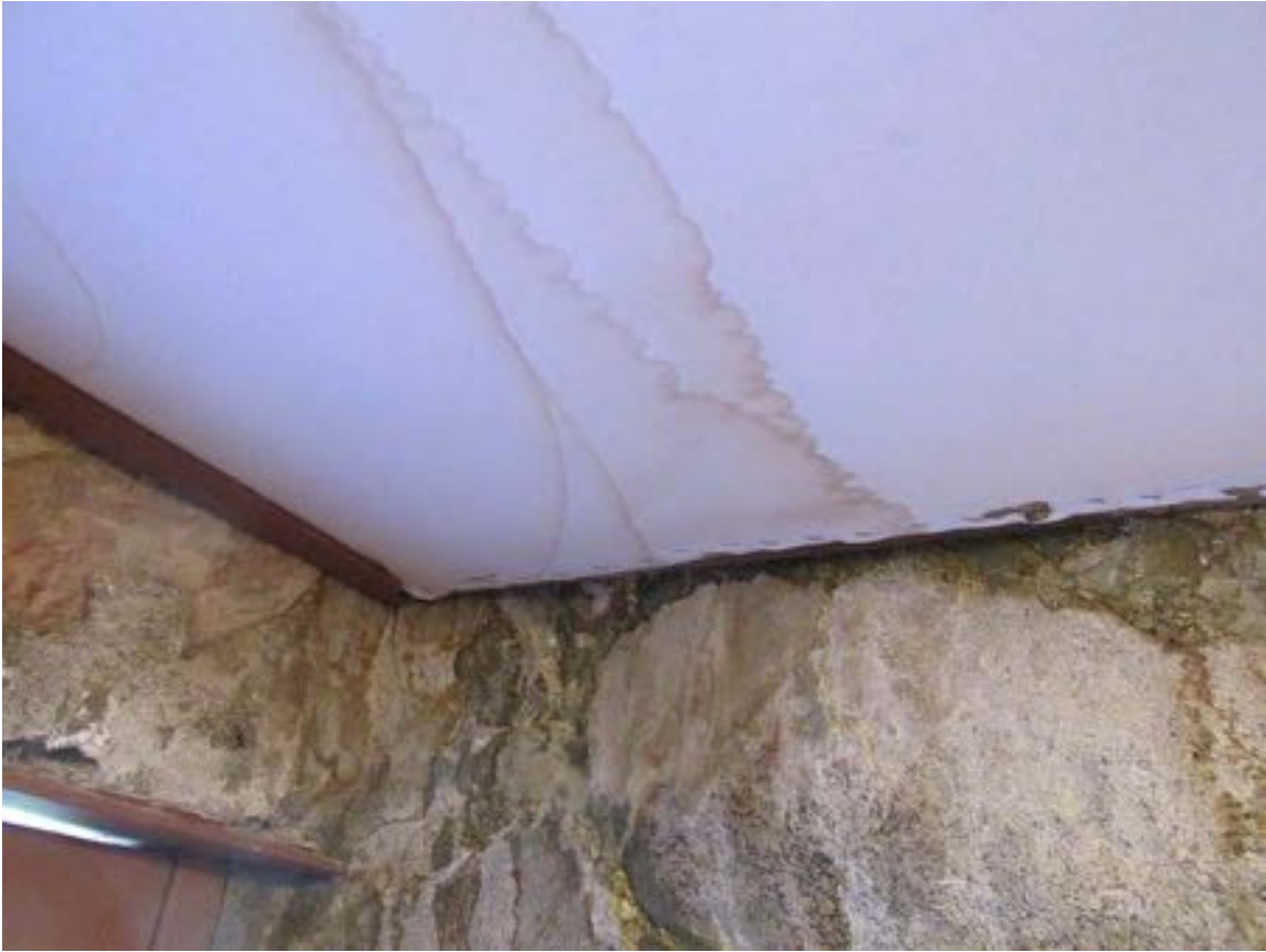
Figure 10-85 - Water stained canvas ceiling in hallway outside the kitchen, 2015 (Harboe Architects).
