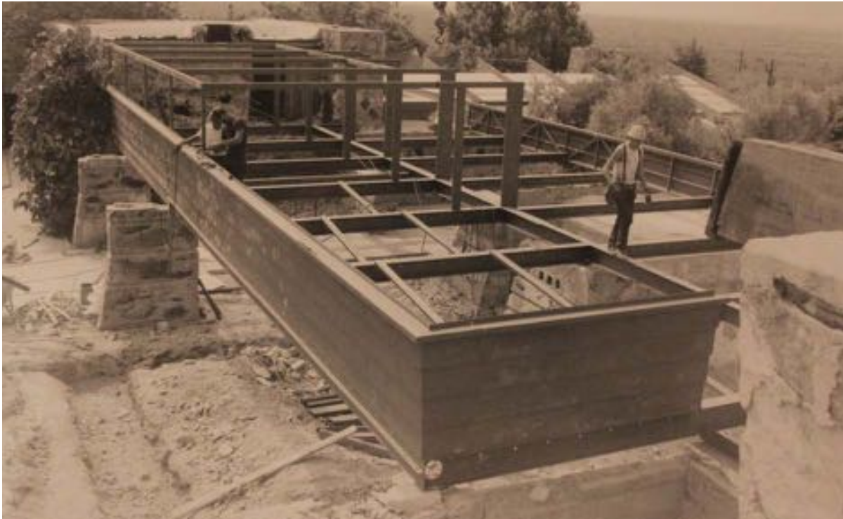
Figure 6-33 - Reconstruction of the Guest Deck in 1970 (The Frank Lloyd Wright Foundation Archives, The Museum of Modern Art | Avery Architectural & Fine Arts Library, Columbia University, New York).
