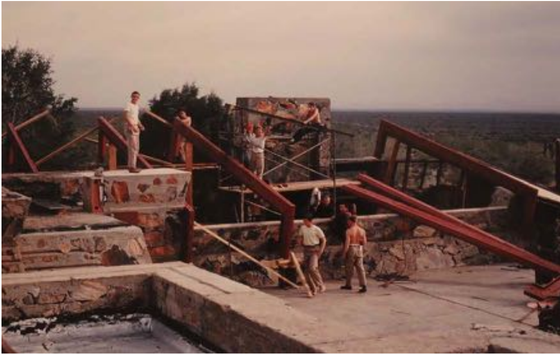
Figure 7-41 - Reconstruction of the Garden Room roof, 1958 (The Frank Lloyd Wright Foundation Archives, The Museum of Modern Art | Avery Architectural & Fine Arts Library, Columbia University, New York).
