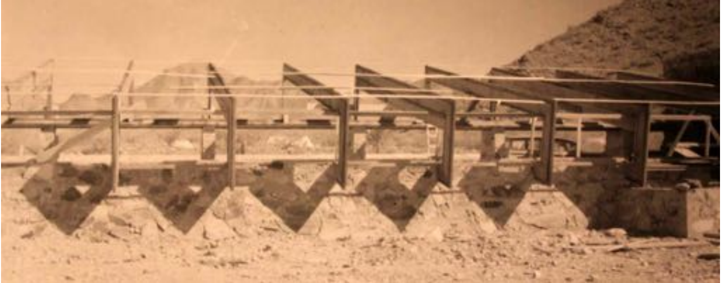
Figure 8-10 - Construction of the Drafting Studio, ca. 1939 (The Frank Lloyd Wright Foundation Archives, The Museum of Modern Art | Avery Architectural & Fine Arts Library, Columbia University, New York).
