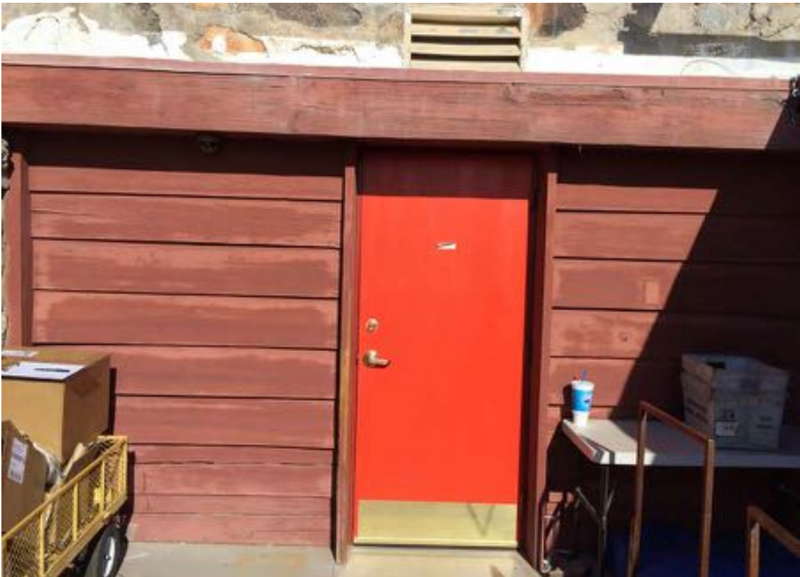
Figure 10-299 - Lap board siding and wood door on west side of Bookstore (Fred Prozzillo).
