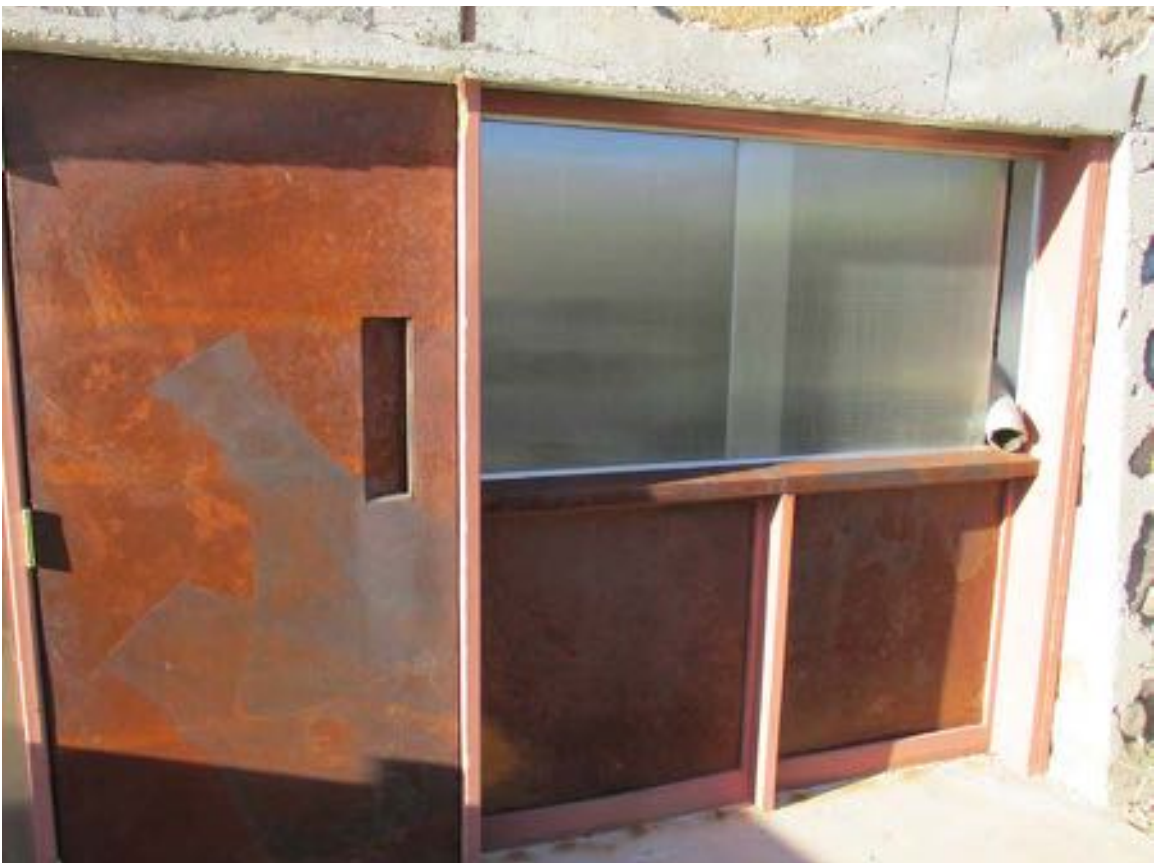
Figure 10-228 - Metal door and glazing on north side of East Wing, 2015 (Harboe Architects).
