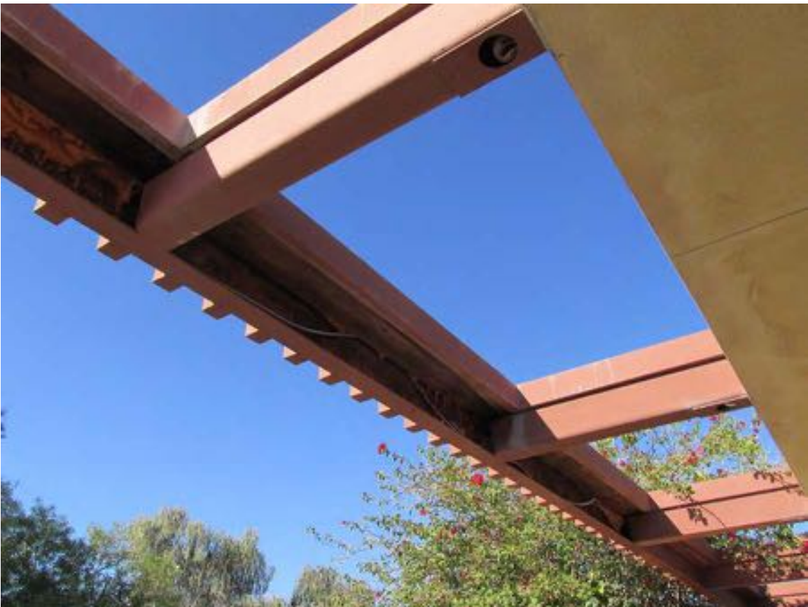
Figure 11-196 - Missing fascia on backside of trellis on south side of the Finance Office, 2015 (Harboe Architects).
