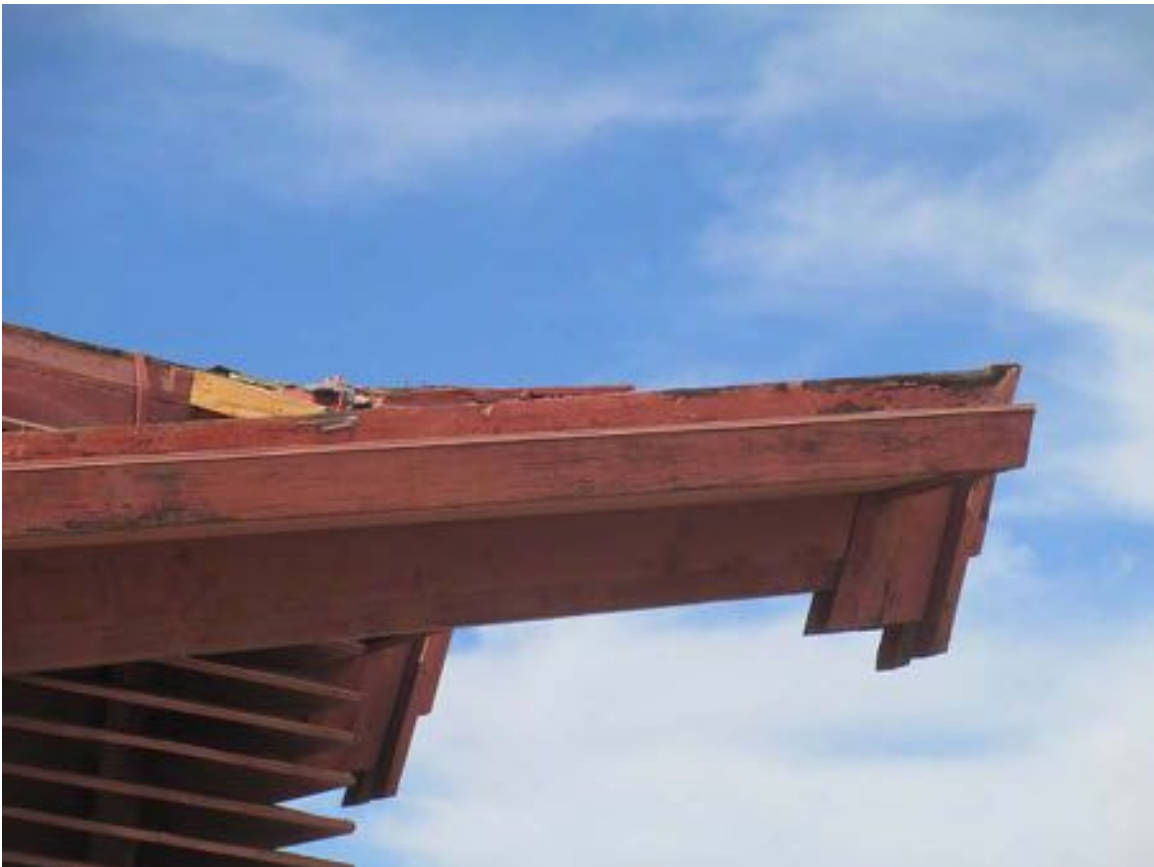
Figure 10-88 - Detail of Water Tower roof showing damaged wood, 2014 (Harboe Architects).
