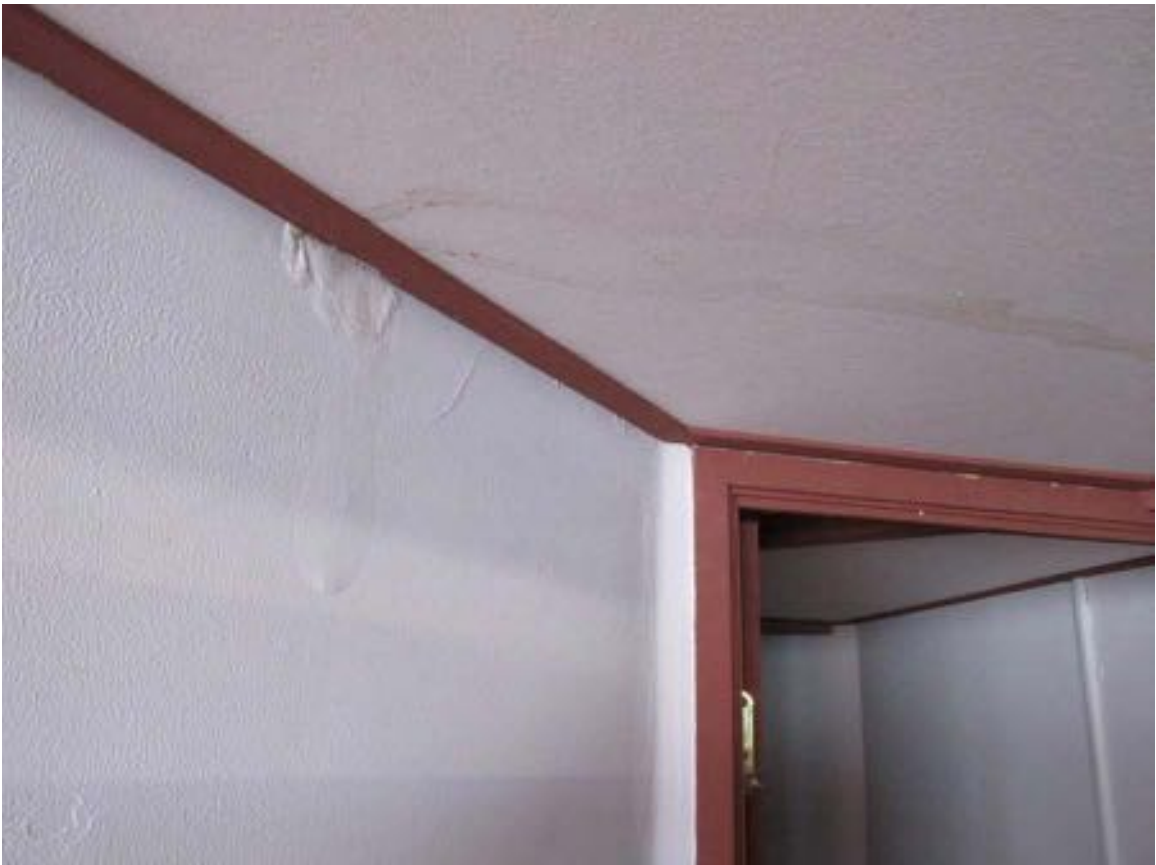
Figure 10-282 - Carney Office showing water damage to wall and ceiling, 2015 (Harboe Architects).
