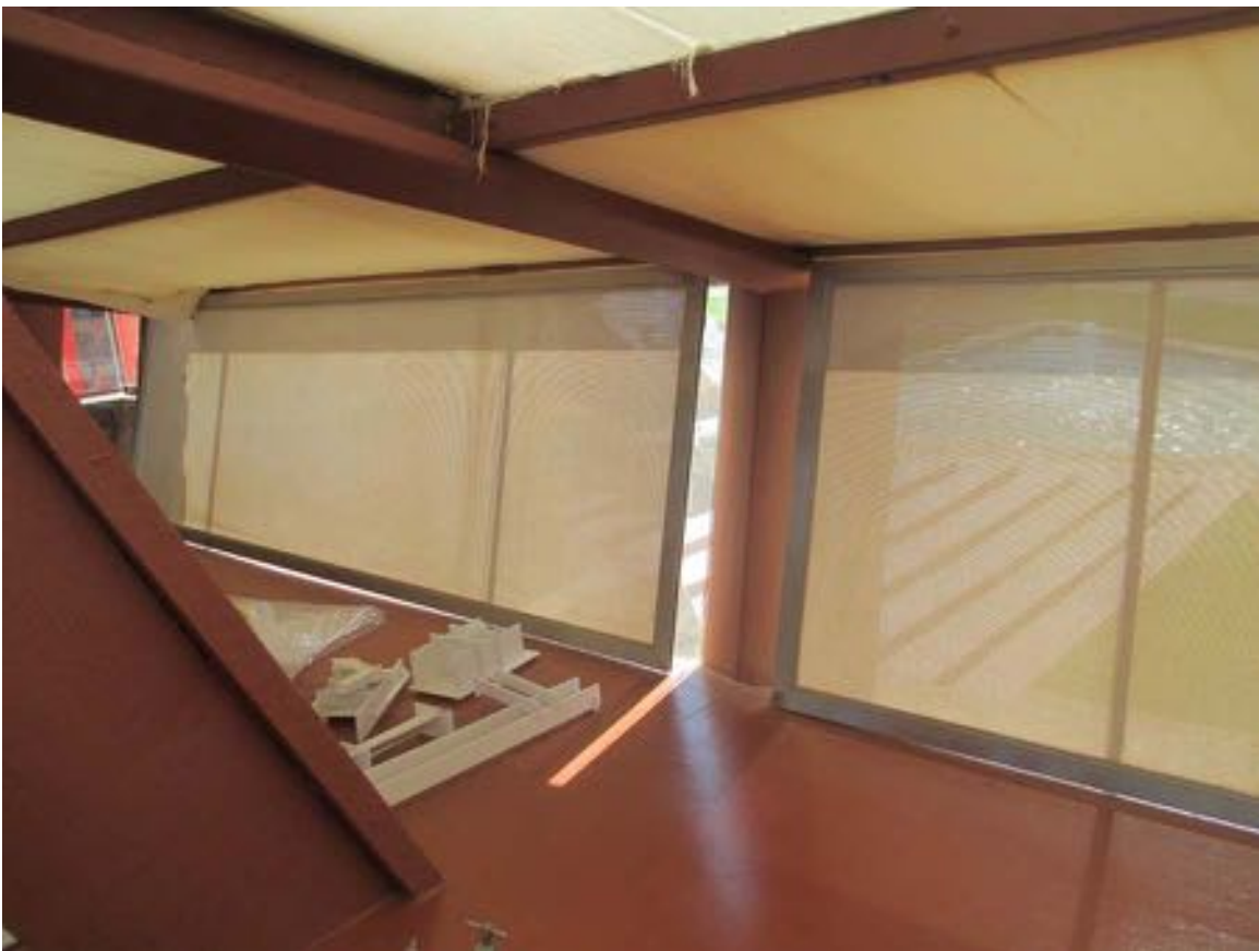
Figure 10-24 - South windows with damaged canvas above, 2014 (Harboe Architects).
