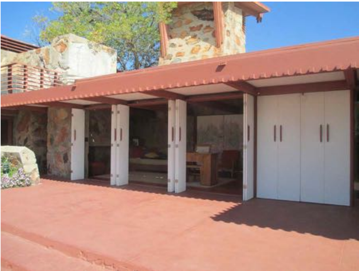
Figure 11-87 - Exterior of Wrights' Living Quarters looking north at wood bi-fold doors, 2014 (Harboe Architects).
