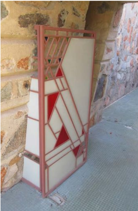
Figure 10-234 - Metal and glass gate at opening to courtyard outside of Finance Office, 2015 (Harboe Architects).
