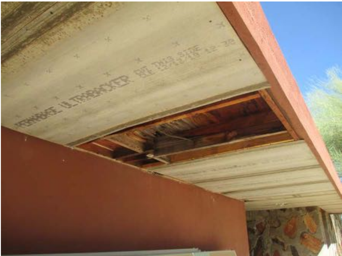
Figure 11-163 - Damaged soffit under flat roof on east side of the Pavilion, 2014 (Harboe Architects).
