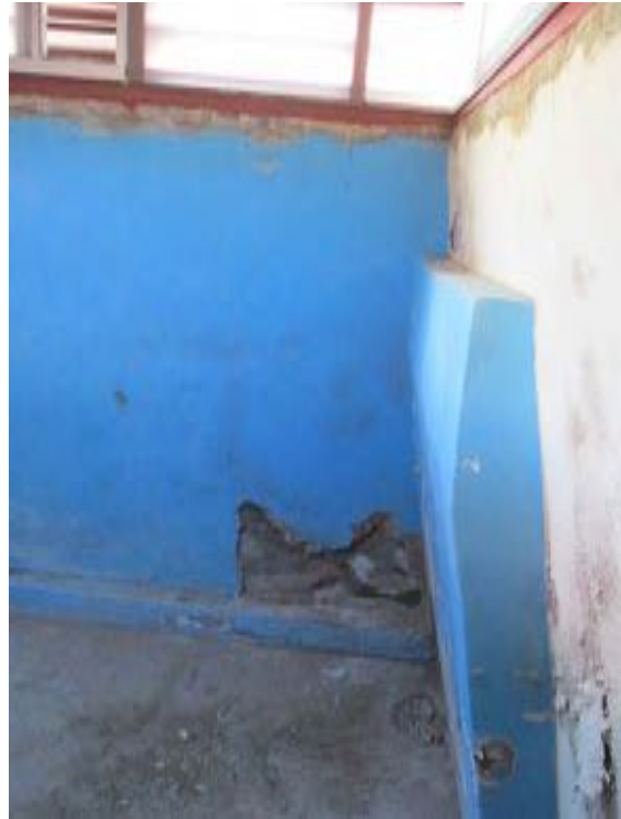
Figure 10-129 - Damaged wall in shower area in Old Men's Locker Room, 2015 (Harboe Architects).
